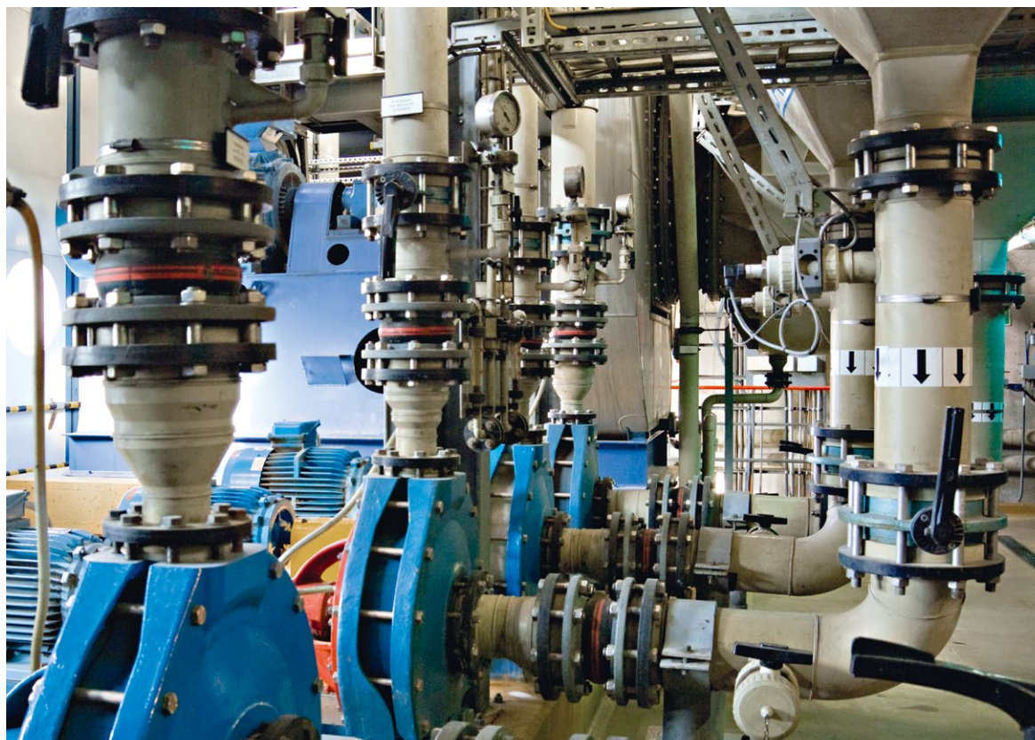
Typical pump station arrangement with expansion joints to decouple pump vibrations from pipeline
