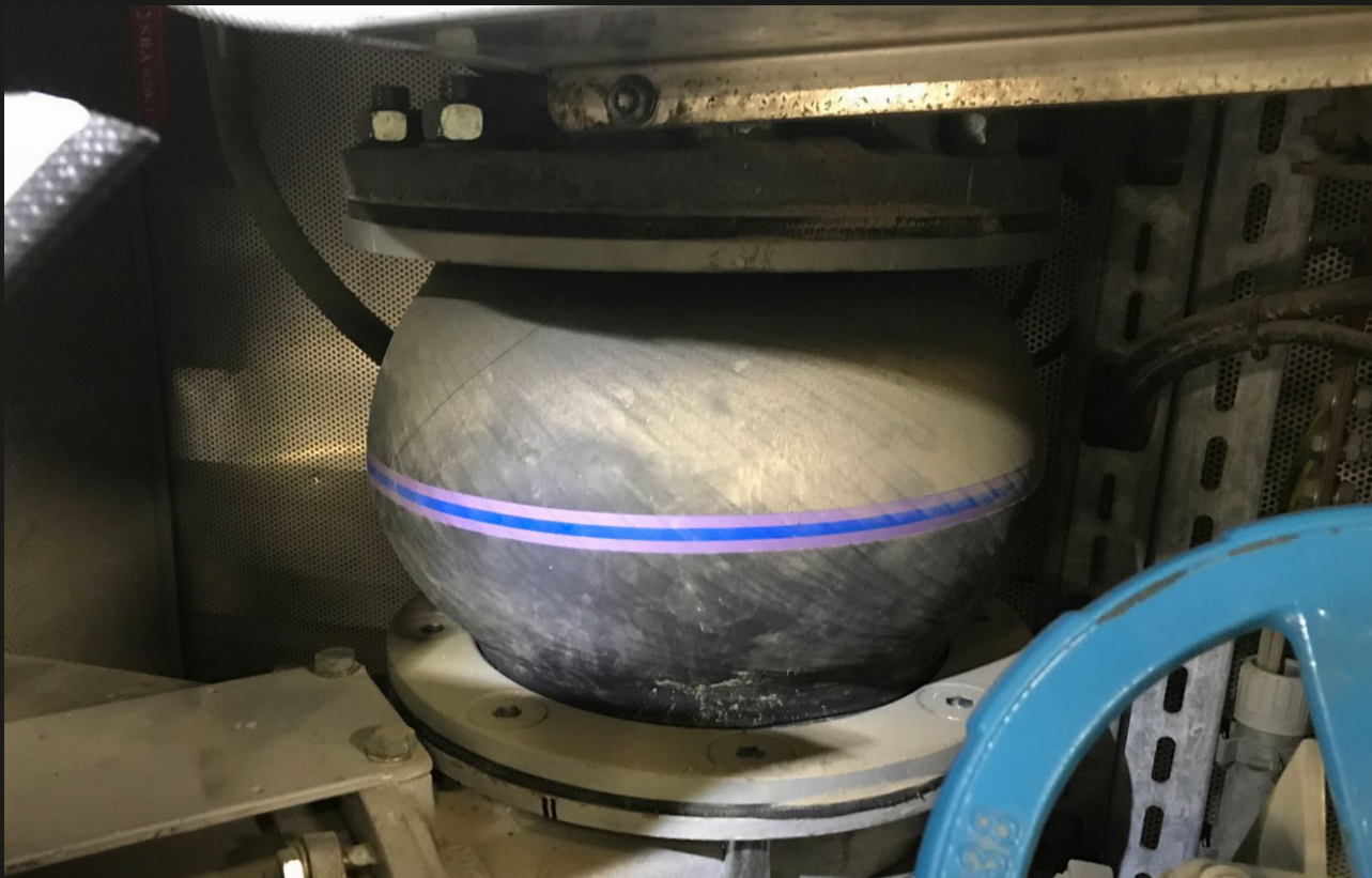
FPM rubber joint Ø 300 mm for 1 bar operating pressure and 180° C, installed on an ash chute
